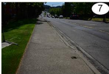
A common situation where a driveway is present in the sidewalk, but does not lead to anything. This situation occurs several times. (photo faces south)
