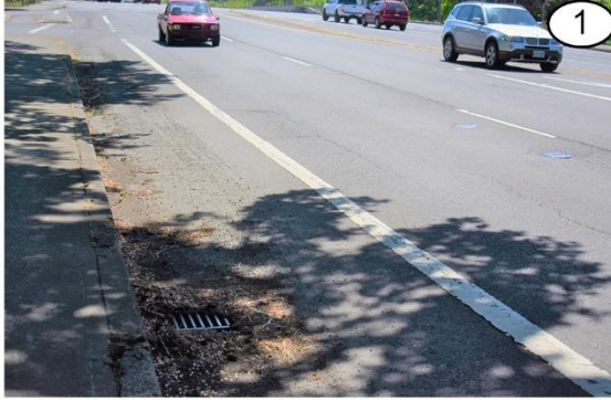
Drainage grates located in bike lane collecting debris. (photo faces north)
