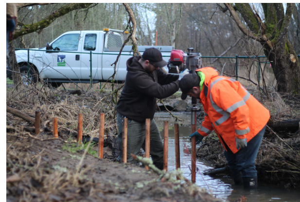
Tigard crew installing light touch grade control using "sticks in the creek"
