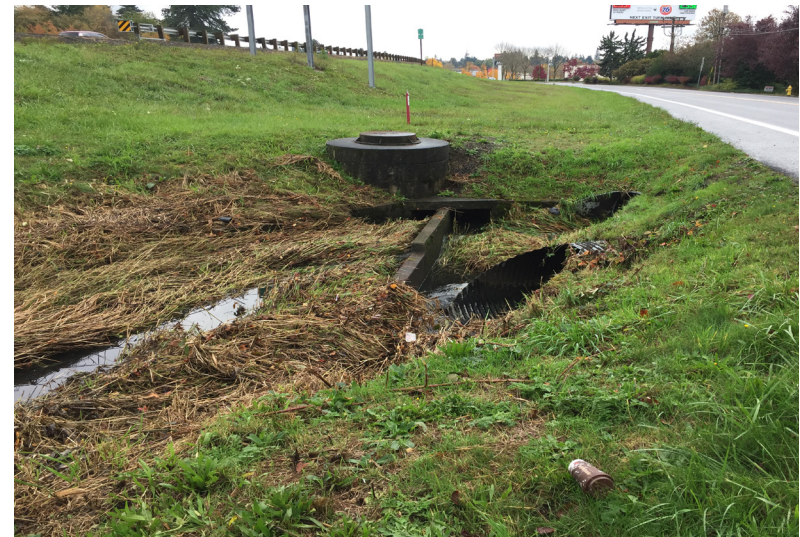
A water quality swale between Hwy 217 and Cascade Avenue treats runoff from the highway
